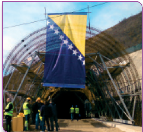
The 2.85 km tunnel, located near Sarajevo, is on highway corridor 5C, which connects central Europe to the Croatian coastline.
